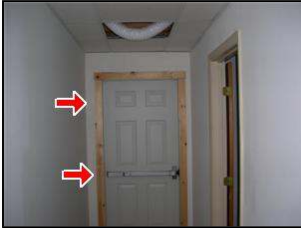
5.3 Picture 1 Cold air/heat loss.
