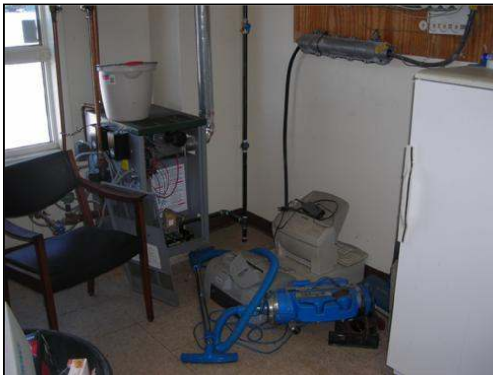
8.0 Picture 1 Service heating system.
