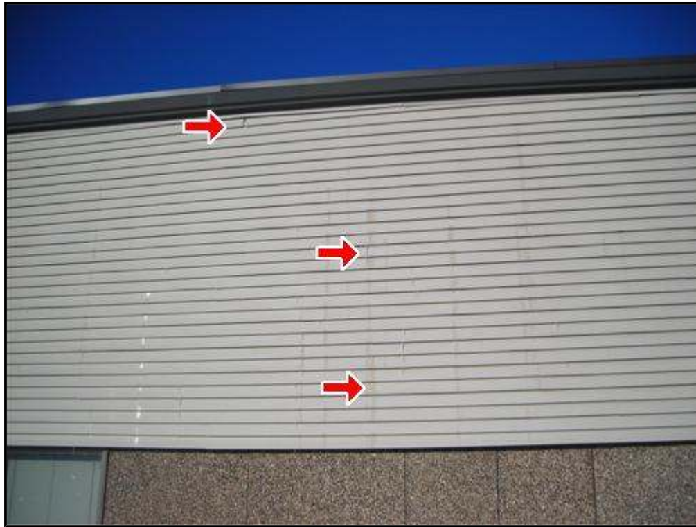
2.0 Picture 1 Moisture intrusion behind siding.
