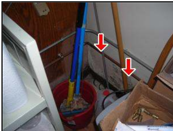
5.1 Picture 1 Moisture penetration.
